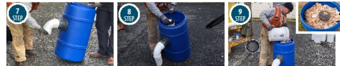
7 STEP Install 4-inch schedule 40 PVC 90-degree elbow downspouts to the threaded nipple.
